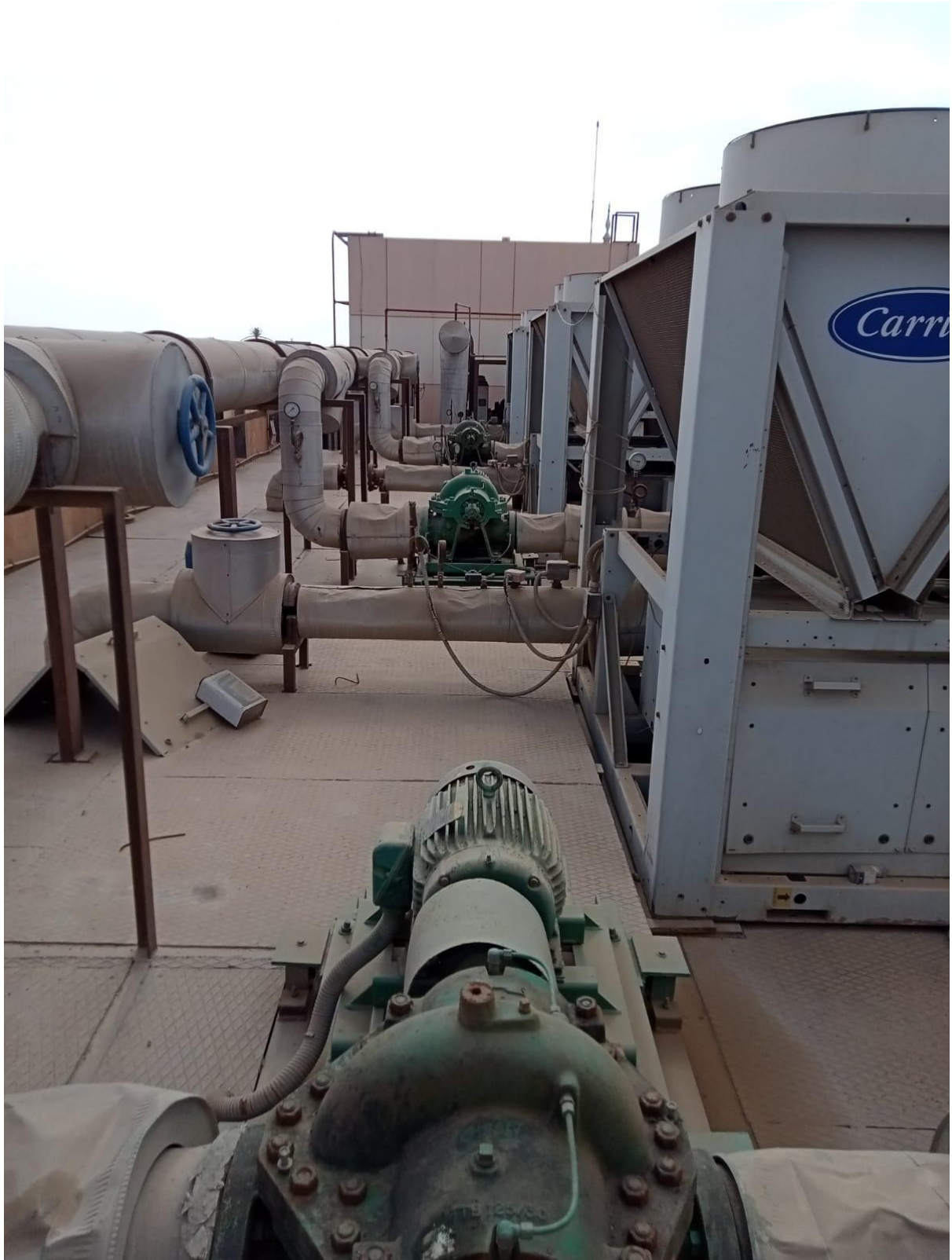
Fig.5. Chillers for the buildings cooling system
