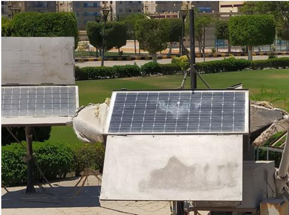
4) Solar Panel in campus
