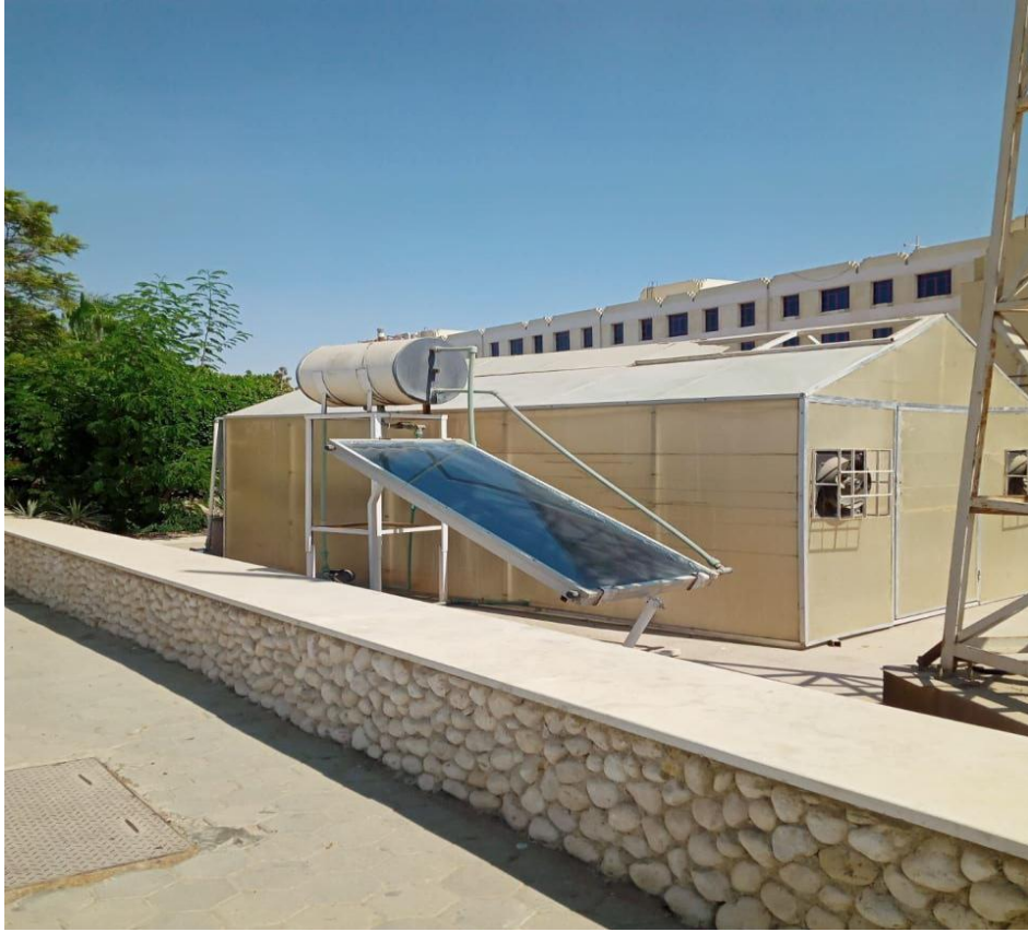
3) Solar water heater
